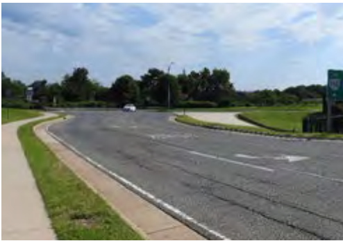
Deteriorating Pavement along Connector Road
