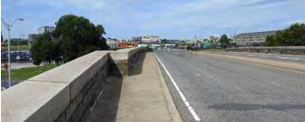
Upgrade Sidewalk Width Deficiency along PTC and Route 110 Bridges
