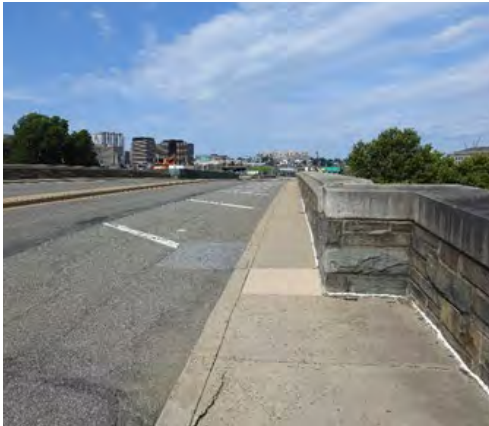
Substandard Sidewalk over Route 110 Bridge
