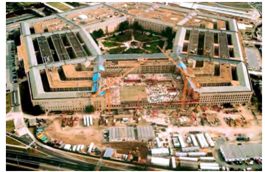
Sections of E, D, and C Rings Removed from West Side for Reconstruction after 9/11 Terrorist Attack, February 6, 2002
