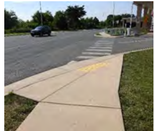
Noncompliant ABA Ramps and Crossing
